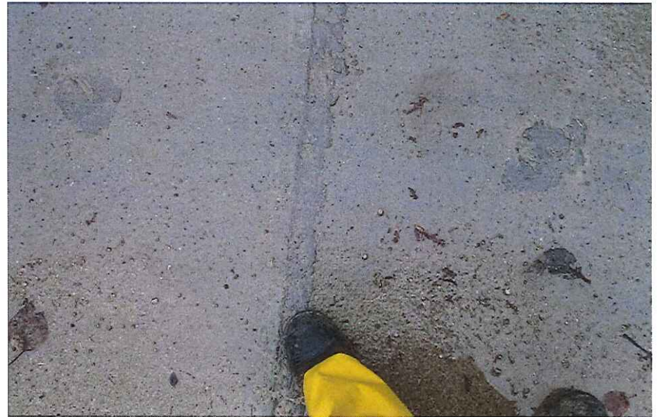
CK2296 Deck Joint
